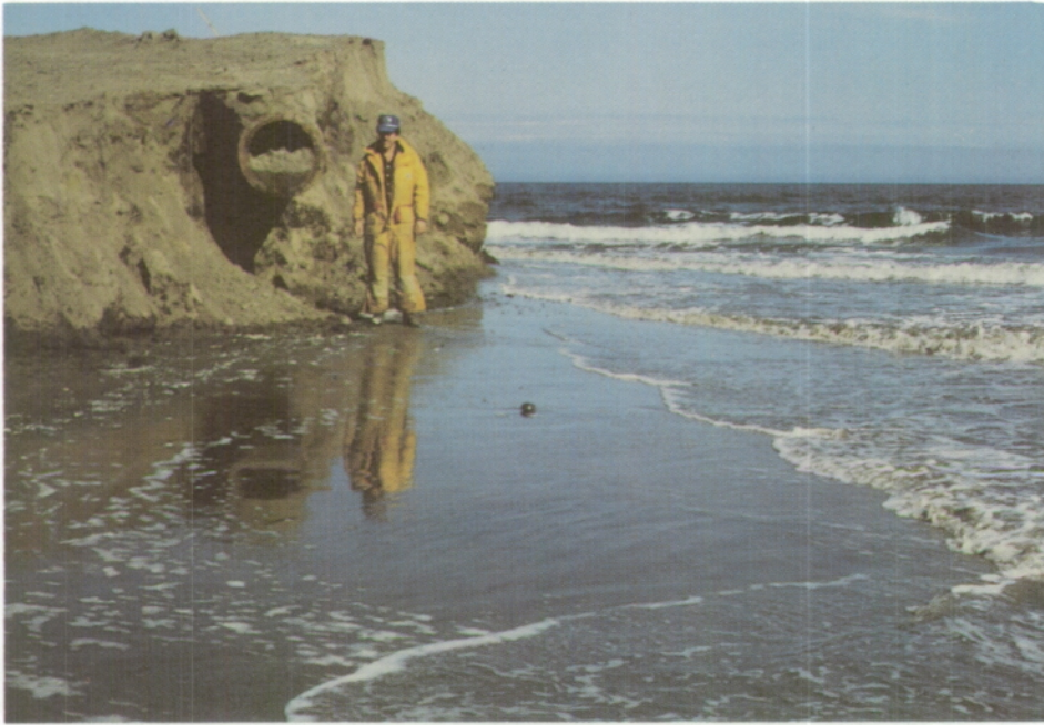
Figure 3.4 Large diameter pipe buried near surface at Profile Line 160, as viewed to the north. (August 10, 1986).
