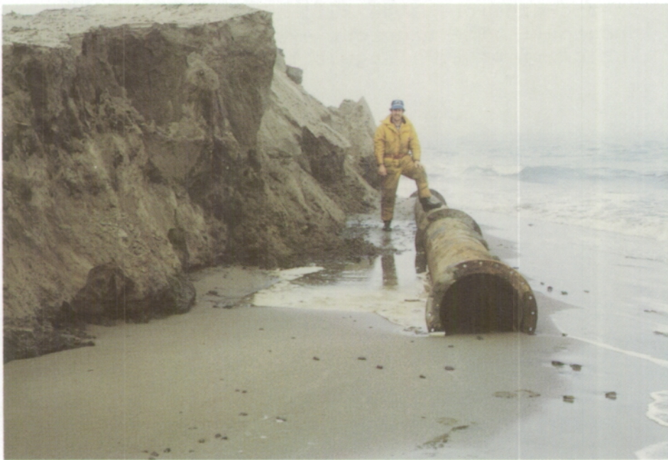
Figure 3.5 Pipe eroded out of cliff at Profile Line 160 two days later. (August 12, 1986).
