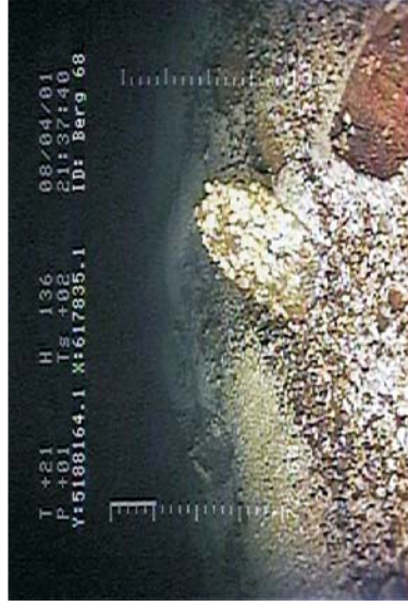
Figure E5: Displaced boulders on the berm
